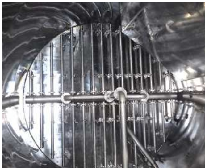
Interior of the salt slurry tank, which has not changed since it went into service (photo taken from above the tank)
