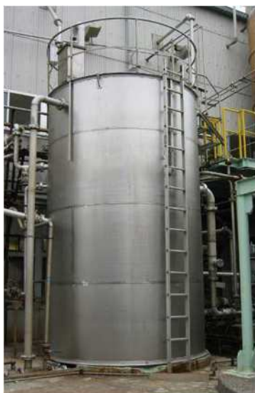
Exterior of the salt slurry tank made from NAS254N steel
