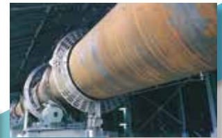
No. 5 rotary kiln (Oheyama Plant)
