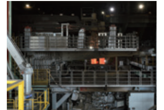
New electric arc furnace ("E furnace")
