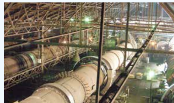
Rotary kiln at Oheyama Plant
