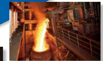
New electric arc furnace ("E furnace")
