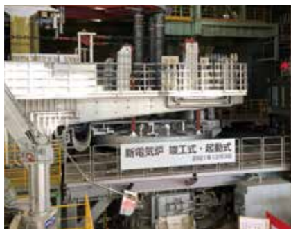
The body of the new electric arc furnace
